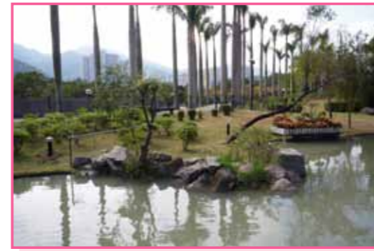
6枝安裝在水池花園的太陽能發光二極管草坪燈 6 sets of solar-powered LED bollards installed in Aviary Garden
