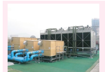
參與廣泛使用淡水於 空調系統的蒸發式冷卻塔計劃 Joined the Scheme of Wider Use of Fresh Water in Cooling Towers for Air Conditioning Systems
