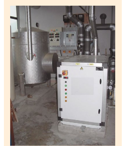
熱泵及儲水箱 Heat pump with water tank
