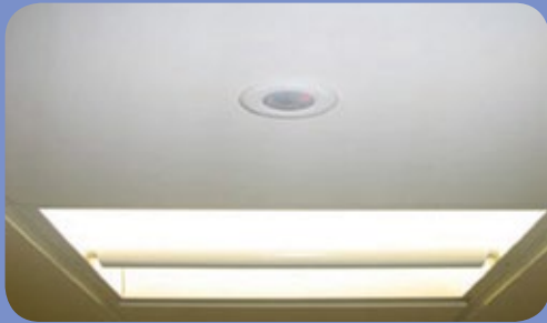
嵌入天花板的用戶感應器 A typical occupancy sensor for lighting control (ceiling mounted)
