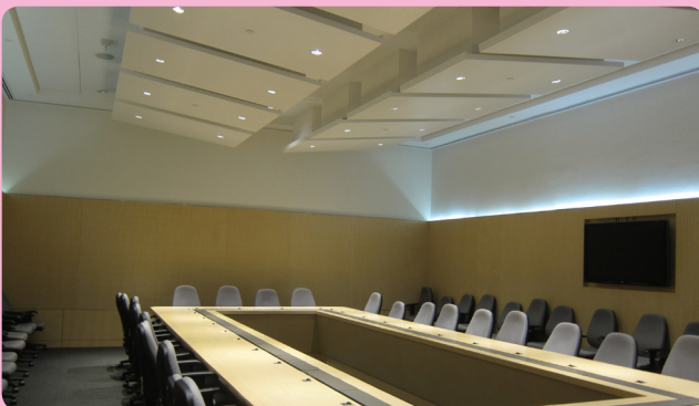
會議室內的LED筒燈 LED down lights at conference room
