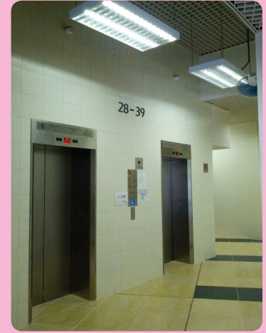
公共房屋項目的LED燈盤 LED lighting panels in Public Housing Project
