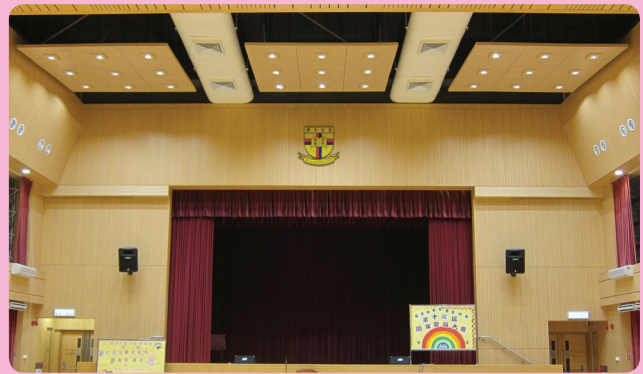
學校禮堂內的LED筒燈 LED down lights in the school hall
