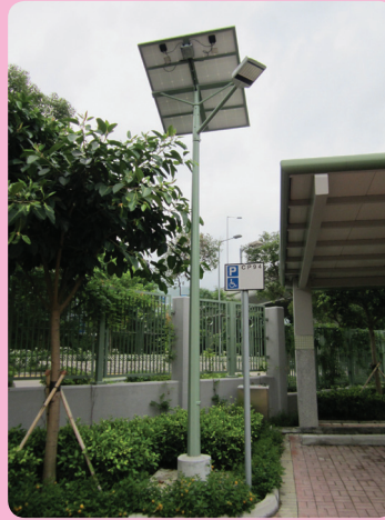
公共房屋項目的太陽能LED燈 LED solar lamp in Public Housing Project
