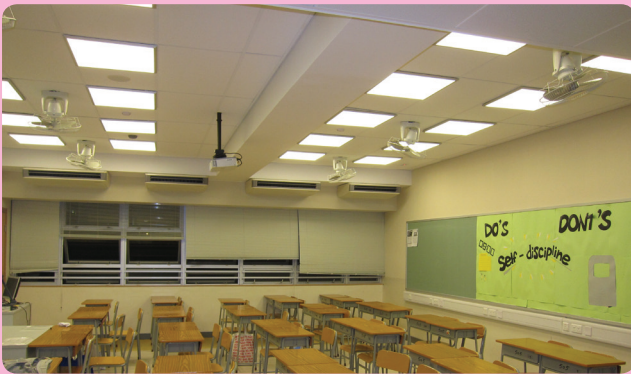
課室內的LED燈盤照明 LED panel lighting at classroom
