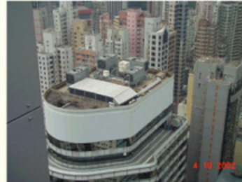
安裝在大有大廈天台的冷卻塔 Cooling towers installed on roof of Tai Yau building
