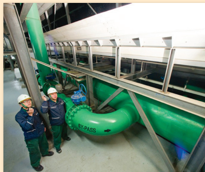
ICC機房內的11米高室內冷卻塔 11m tall indoor cooling towers inside the ICC plant room
