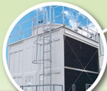
空調裝置 Air-conditioning installation
