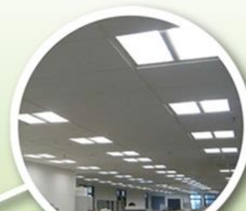
照明裝置 Lighting installation
