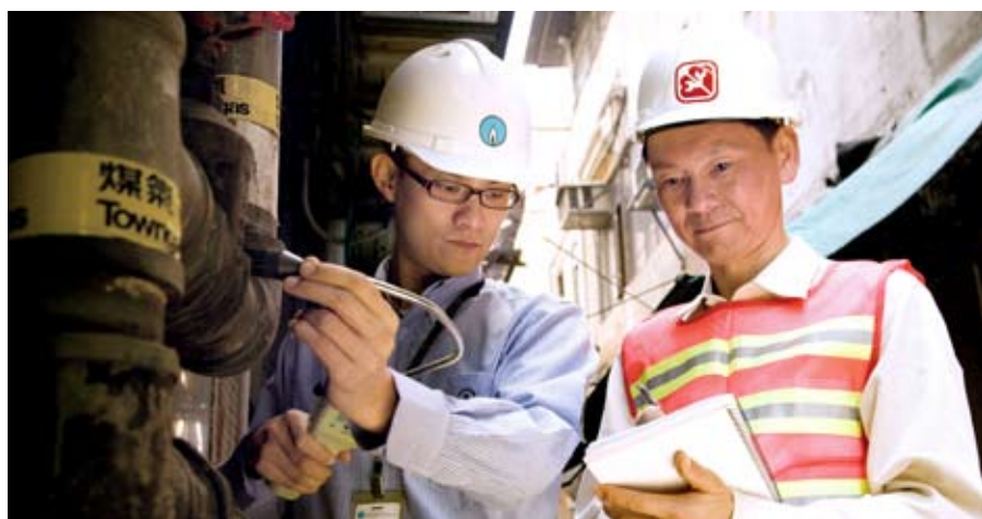
Increased inspections have significantly reduced gas riser incidents.
