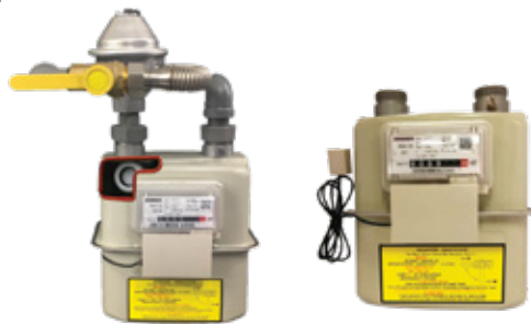
Figure 4: Smart Gas Meter installed in a Kitchen of a Local Domestic Premises
