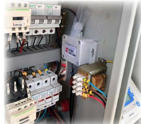
位於圓洲角診所監測冷氣系統的感測器 Dry contact sensor installation for air-conditioning system at Yuen Chau Kok Clinic
