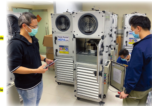
機電署同事為普通病房安裝「流動組合式 - 高效能空氣微粒子過濾器」把其改裝為負壓病房 EMSD colleagues converting general wards into negative pressure wards by installing MMHU
