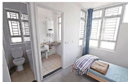
檢疫隔離中心內的機電設備 E&M equipment at a quarantine centre
