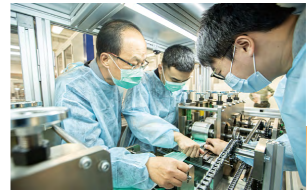
為懲教署裝設口罩生產機 Installation of mask production machines is carried out for the CSD
