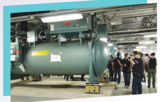
特定機電團隊(暖通空調)實地考察港珠澳大橋海水泵房原型 The SDU (HVAC) undertook a site visit to the prototype of the seawater pumping facility of the Hong Kong-Zhuhai-Macao Bridge
