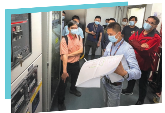
特定機電團隊(電力)參觀屯門醫院總掣房和了解流動發電機供電轉掣的程序 The SDU(E) visited the main switch room of Tuen Mun Hospital and learnt about the procedures of power switch of the mobile generator
