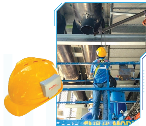
機電署在區域供冷系統工程採用智能安全帽，以提升工地安全 The EMSD has adopted smart helmets in the District Cooling System Plants to enhance site safety
