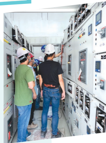
機電署與建造團隊緊密合作，日以繼夜進行測試工作，務使香港感染控制中心順利投入服務 In close collaboration with the construction team, the EMSD staff worked round-the-clock to conduct tests to ensure the smooth commissioning of the HKICC
