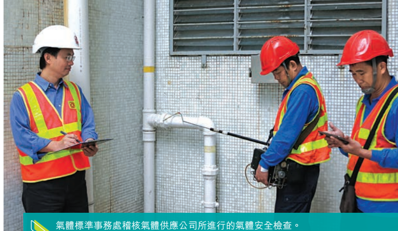
▶ 氣體標準事務處稽核氣體供應公司所進行的氣體安全檢查。 Gas Standards Office auditing the gas safety inspection work being carried out by a gas supply company.
