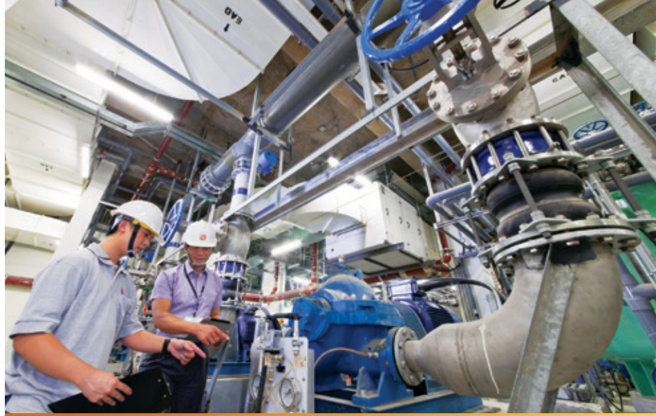
我們的專業人員為新屯門西北游泳池的過濾系統進行定期檢查。 Our professional staff is conducting regular inspection of the filtration system at the new Tuen Mun North West Swimming Pool.
