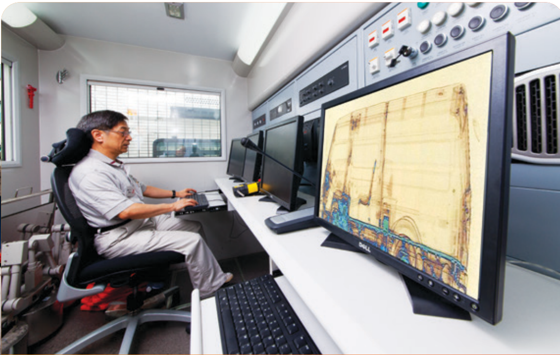
營運基金工程師正在測試用作監控掃描過程和實時檢視掃描影像的精密儀器。彩色 X 光影像可清楚顯示被掃描車輛內的不同物料。 An EMSTF engineer is testing the sophisticated equipment for control and monitoring of the scanning process and real time image display. A colored x-ray image shows clearly different materials in the scanned vehicle.
