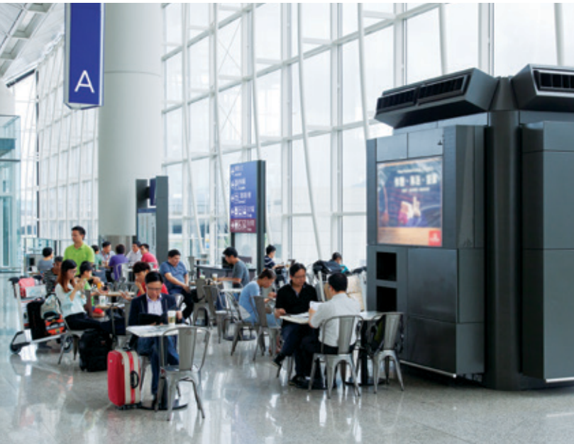
我們維修保養機場空調系統，為旅客提供舒適環境。 We maintain the airport air-conditioning system to give travellers a comfortable environment.
