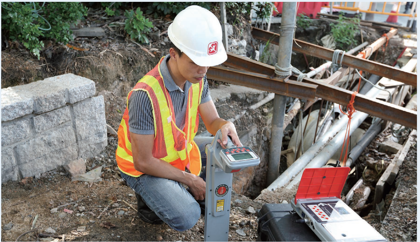
機電工程署員工到工地巡查，確保第三者工程不影響供電電纜安全。 EMSD staff inspect worksites to make sure electricity supply lines are safe from third party works.
