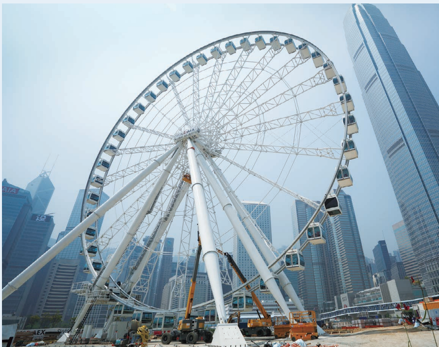
中環海濱摩天輪項目逐漸成形。我們會先進行各項檢查和測試，才發出使用批准。 The Hong Kong Observation Wheel by the Central waterfront is taking shape. We shall conduct inspections and tests before granting approval for its opening.
