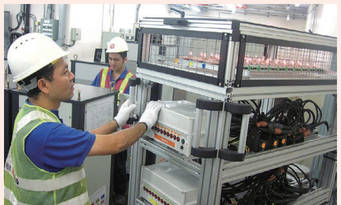
我們的維修團隊與香港機場管理局，共同設計一套固定電流調節器測試平台，並取得專利。測試平台可在室內快捷地測試機場跑道燈，減少對跑道運作的影響。 Our maintenance team jointly designed and patented the Constant Current Regulator Testing Platform with the Airport Authority Hong Kong, allowing us to test the airfield ground lighting indoor and work faster, minimising disruption to runway operations.
