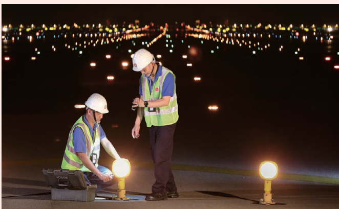
我們為超過10 000盞機場跑道燈提供專業的維修服務，確保飛機於跑道及滑行道可安全升降和行駛。 We provide professional maintenance services to over 10 000 airfield ground lightings, ensuring runways and taxiways are safe for taking-off, landing and manoeuvring of planes.
