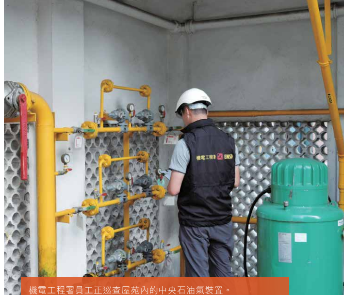
機電工程署員工正巡查屋苑內的中央石油氣裝置。 EMSD staff inspecting an LPG central supply installation in a housing estate.
