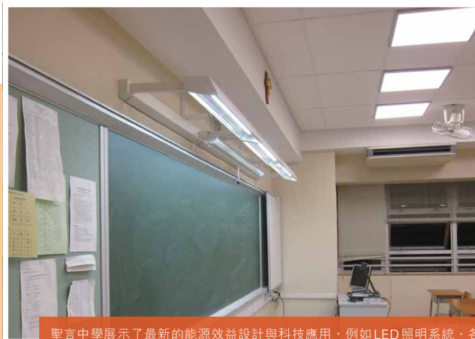
聖言中學展示了最新的能源效益設計與科技應用，例如LED照明系統、各種可再生能源裝置、及全港首個在學校使用的淡水水冷式中央空調系統。 Sing Yin Secondary School features state-of-the-art energy efficiency designs and technologies, such as LED lighting, various renewable energy installations as well as a fresh-water-cooled centralised air-conditioning system, the first in a school setting.
