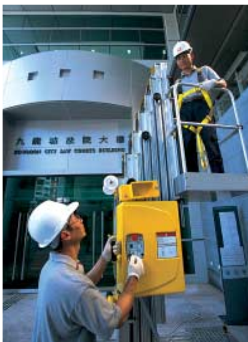
技術人員在九龍城法院大樓維修照明系統。 Technician repairing the lighting system at the Kowloon City Law Courts Building.
