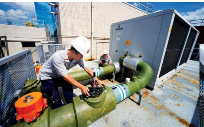
我們定期檢查空調系統，確保運作正常。 We conduct regular checking to ensure the air conditioning system is under normal working condition.
