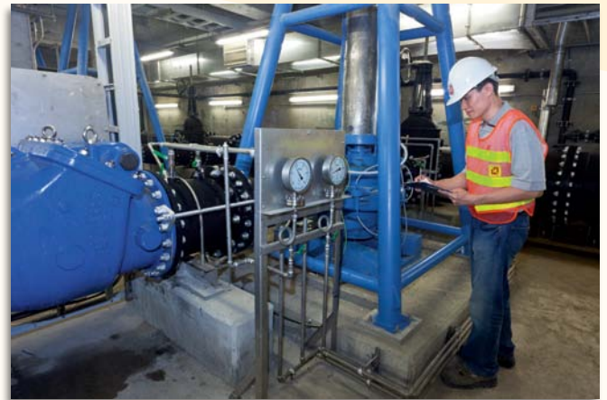
中環填海工程第三期的海水泵房設施主要服務添馬艦新政府總部的空調系統。 Seawater pumping facilities at the Central Reclamation Phase III Seawater Pump House are mainly used for air-conditioning systems at Tamar.
