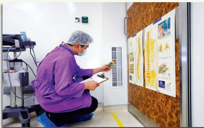
為香港佛教醫院的手術室機電系統進行測試及校驗，確保符合嚴格標準。 Testing and commissioning is being conducted on the E&M systems in the operating theatre of the Hong Kong Buddhist Hospital to ensure their compliance with relevant stringent standards.
