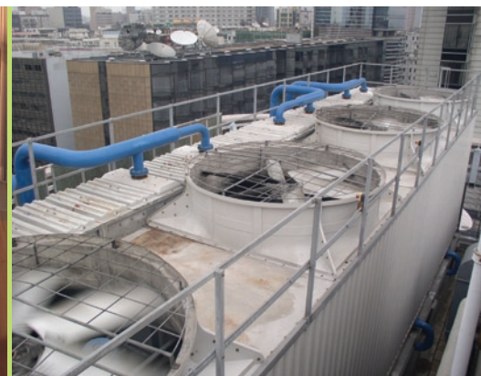
Water Cooling Towers at Young Men's Christian Association, Tsim Sha Tsui
