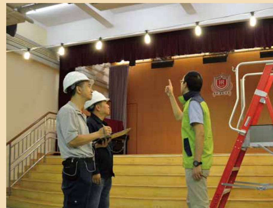
我們的同事為各投票及點票站安裝額外照明設施，並進行檢測工作。 Additional lightings were installed at the polling and counting stations and inspected by our staff.
