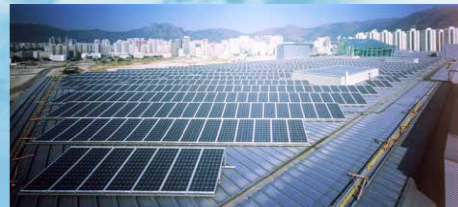
機電署總部大樓安裝了全港市區內最大型的太陽能光伏系統。 EMSD Headquarters Building is installed with the largest Photovoltaic System in Hong Kong urban area.
