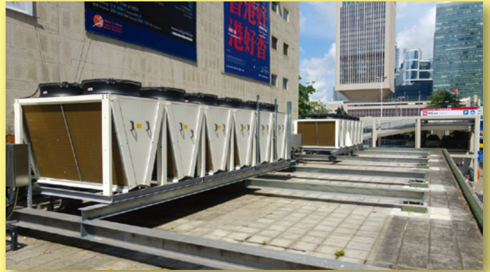
遠距冷凝系統的風冷式冷凝機組安裝於大會堂低座天台，作為應急方案的一部分。As part of the contingency plan, the air-cooled condensers of the remote condensing system are installed on the rooftop of the City Hall Low Block.
