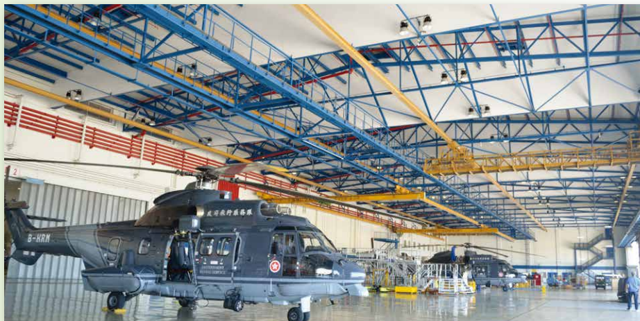
我們為政府飛行服務隊總部飛機庫安裝的線式熱力感應器可靠耐用，特別適合通風的開放式環境。 The linear heat detectors installed in the hangar of the GFS Headquarters are reliable and durable, especially fit for open and ventilated environment.
