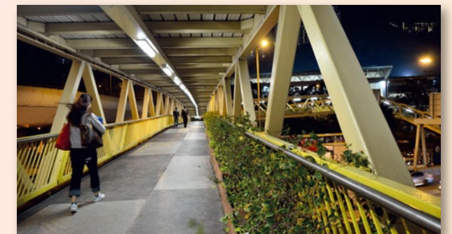
我們率先在彩虹斧山道橫跨龍翔道的行人天橋裝設新的「智能調光照明控制系統」，安裝後用电量較以往節省多達50%。 The new Smart Footbridge Lighting Dimming Control System was first installed at the footbridge at Hammer Hill Road, Choi Hung, across Lung Cheung Road. The electricity consumption was then saved by as much as 50%.
