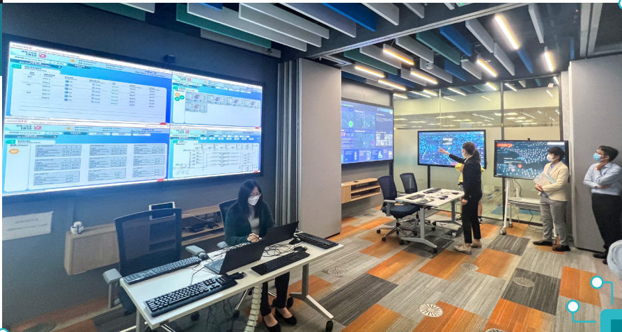
機電署人員會利用綜合樓宇管理系統為入境處新總部提升日常管理效能。 The EMSD staff will utilise the iBMS to enhance day-to-day management efficiency of the new Immigration HQ.
